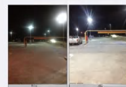
XJ-FL100W Flood Light in Australian Parking Lot
