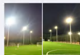
XJ-FL Flood Light in Football Field, Dubai
