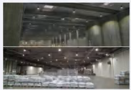
XJ-HBK130W Highbay in warehouse, Denmark
