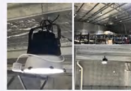
XJ-HBS200W Highbay with sensor in Austria warehouse.
