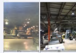
XJ-HBG150W replace 400W MH in Germany
